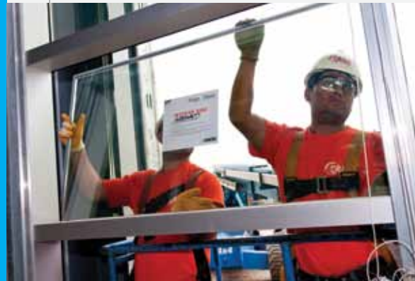
Sage glass, being installed at the Siemens - US Nacelle Facility in Hutchinson, Kan., is designed for energy efficiency.
