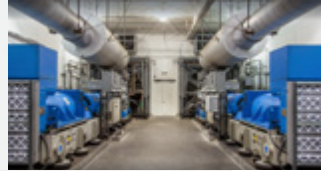
Digital Realty's 365 Main data center in San Francisco, CA. Digital Realty Trust is the world's largest wholesale data center provider.
